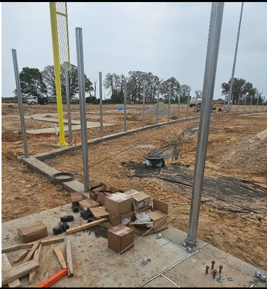
Baseball entrance needs to be wider for a double gate
