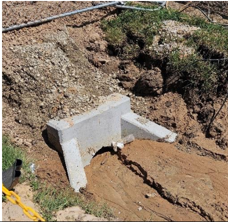
Culvert completely blocked by silt
