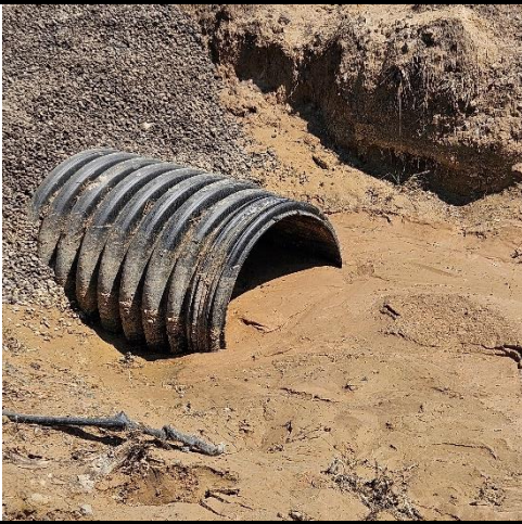
Ditch Culverts blocked by erosion
