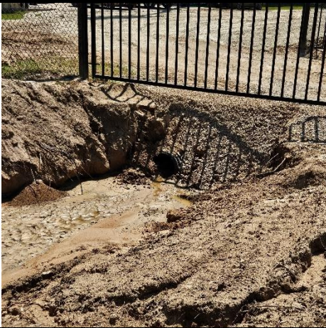
Culvert blocked by silt
