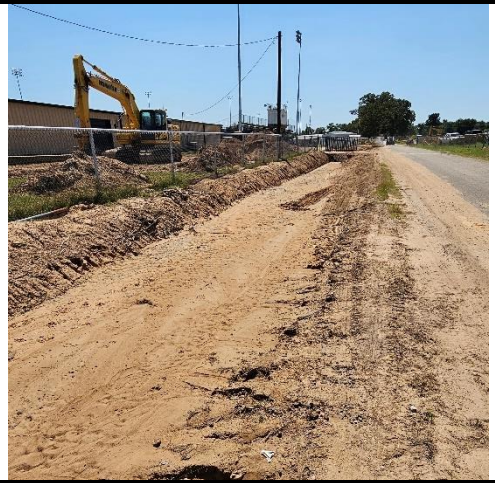
Ditch needs to be re-graded and grass in place
