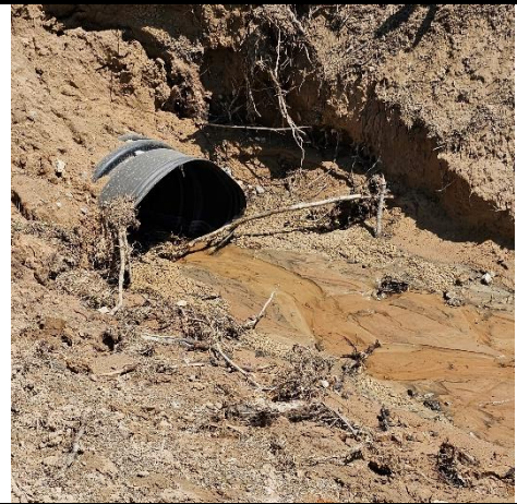
Culvert blocked by silt
