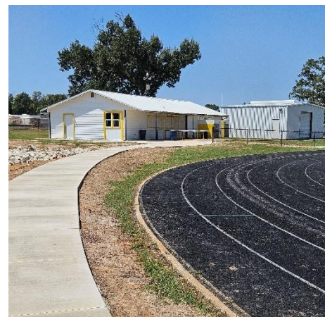
Endzone sidewalk, grass needed and new fence to be installed
